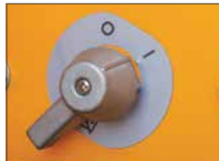
BATTERY DISCONNECT SWITCH
