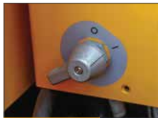
BATTERY DISCONNECT SWITCH
